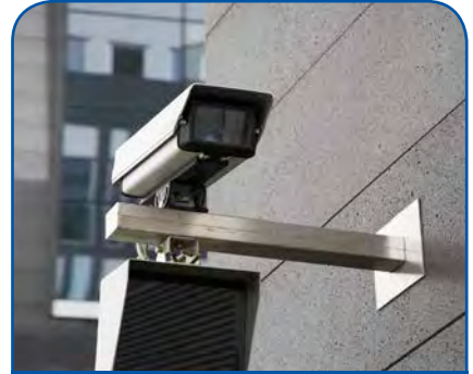
Building Automation & Control
