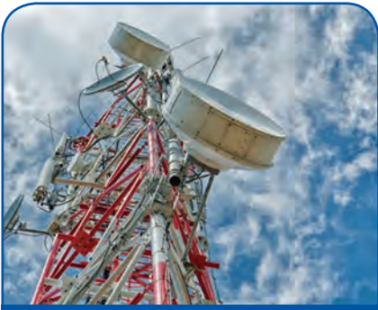
Telecom -Data Infrastructure
